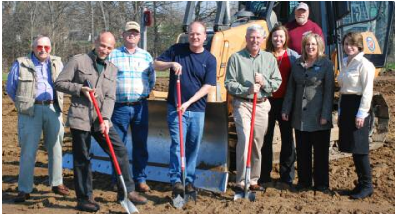
Pictured at the groundbreaking ceremony for the solar array Thursday morning are: Village Councilman Lynn Miller, SP&L representative Brett Henderson (a St. Paris native), Village Administrator Joe Sampson, Village Mayor Joe Braden, village economic development consultant Dave Faulkner, Champaign County Chamber of Commerce representative Andrea Tullis, Chamber of Commerce Director Tina Knotts, Dovetail Regional Sales Manager Siobhan Pritchard and John Haulman of Champaign Excavating (on the tow plow in back).
